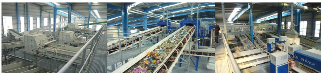
Figure 2: Material Recovery Facility at Nafkias, Kochi Community, Region of Larnaca CYPRUS
